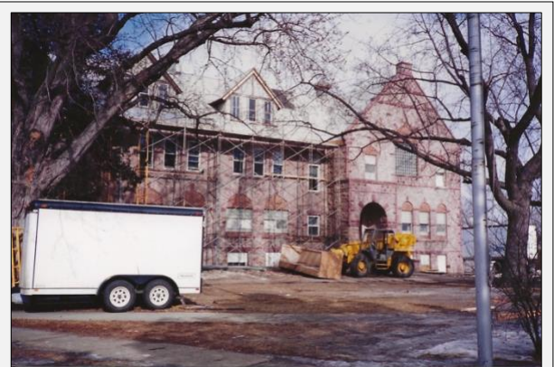
By the late 1990s, the Olde School was being renovated into apartment housing, beginning a new chapter of community use after years of dormancy.
