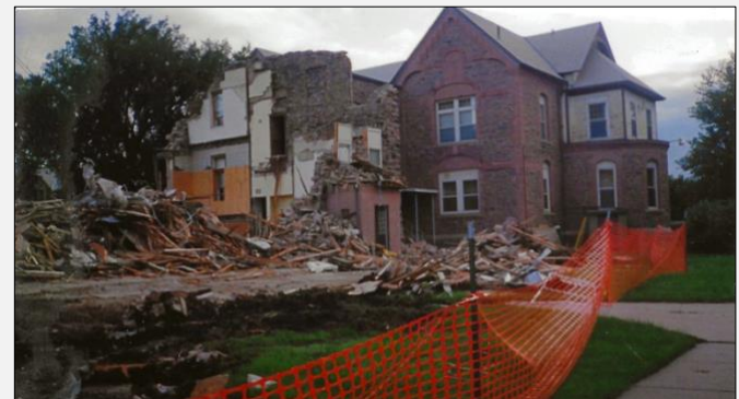
Demolition of French Hall in 1993, marking the end of a long-standing part of the campus history and decades of memories for the SDSU community.
