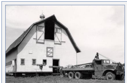
The main SDSD farm barn being relocated in 1949 to the east side of Sioux Falls, near Sycamore Avenue and 6 th Street. The structure remained in use until it was removed in the 1990s for construction of Washington High School.
